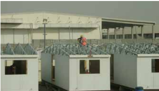
MIDDLE EAST - Modular Units
